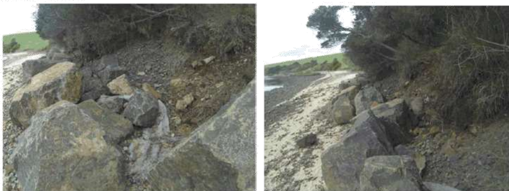
Erosion of rock revetment SE of James Oates Reserve boat ramp
