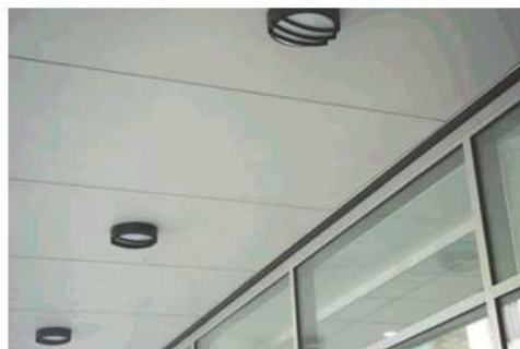
Bunker lights are a simple, cost effective and vandal resistant option for under awning lighting
